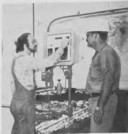
Job leader Patricio Kock observes how Bob Aronson installs explosion-proof flowmeter at Finger Pier No. 1.
